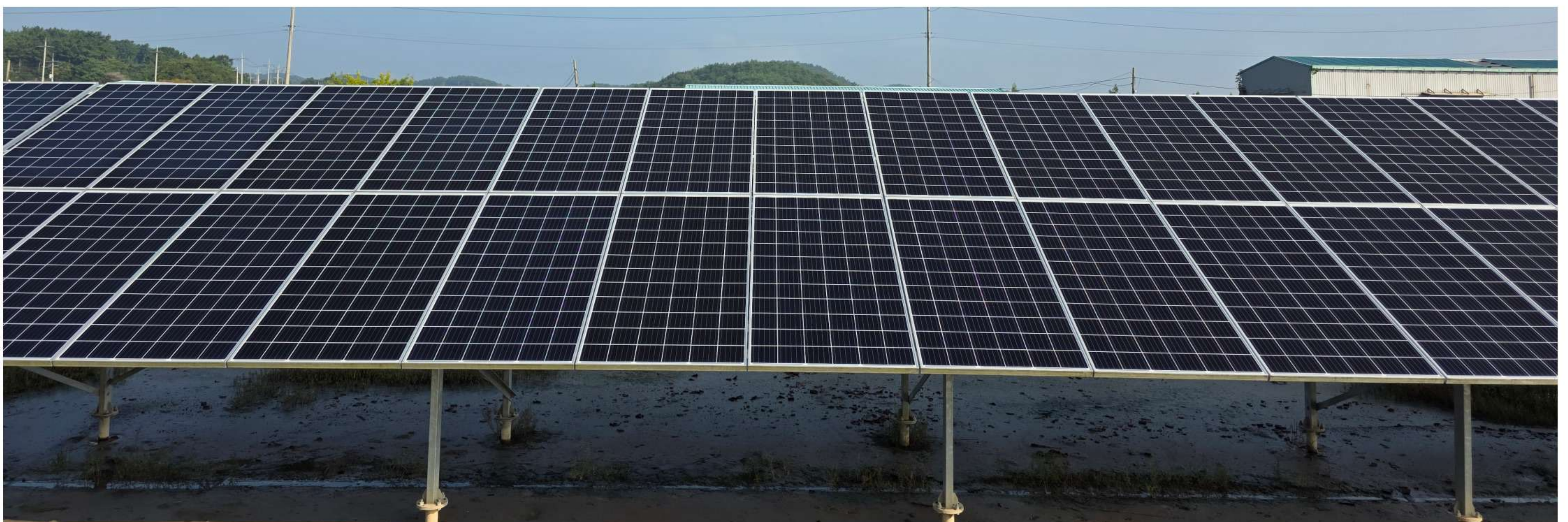
Solar PV asset in South Korea
