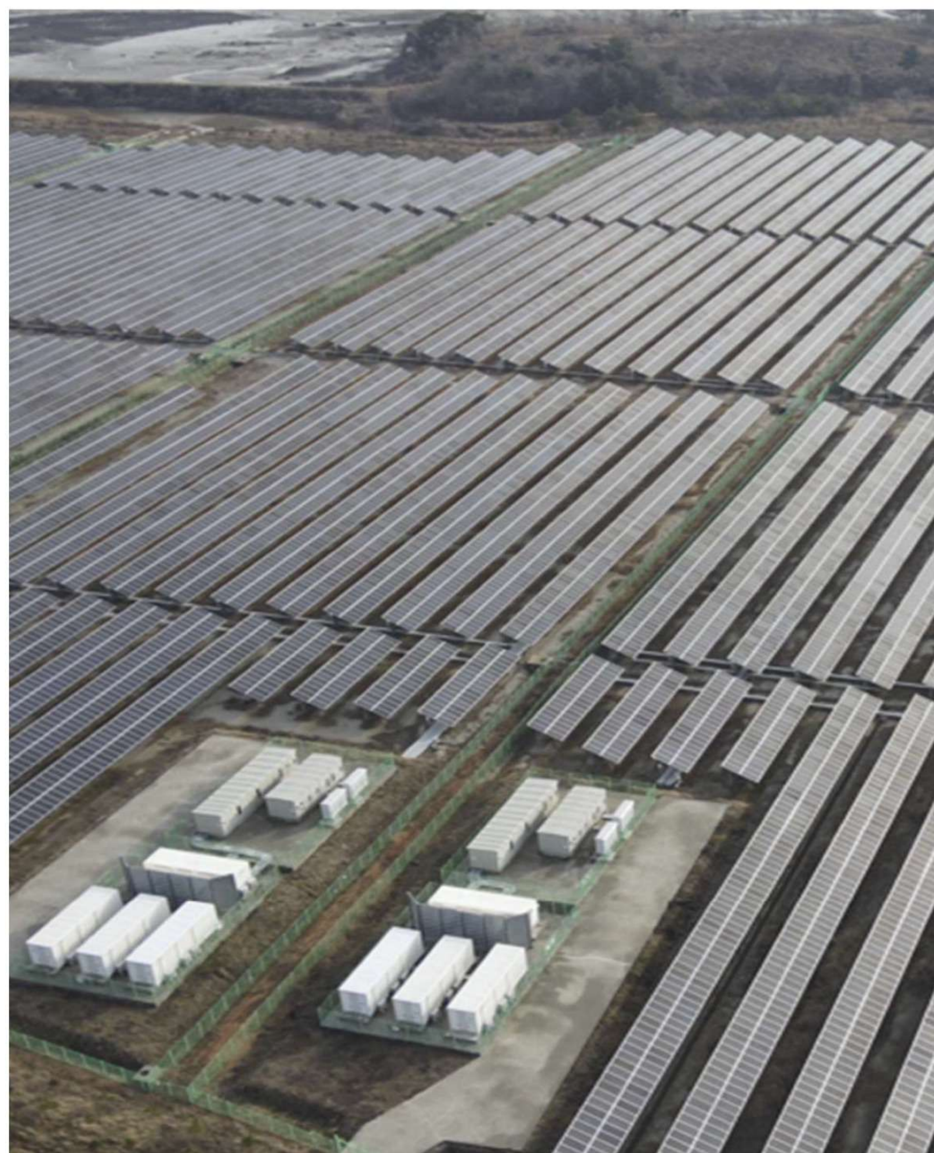
Solar PV and battery storage asset in South Korea
